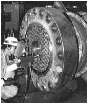
The tube-to-tubesheet joint of a heat exchanger made of heat resistant steel is TIG welded by using an orbital welding machine and filler metal.
