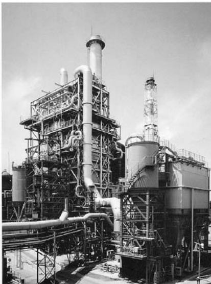
Figure 1: A coal-fired steam boiler consisting of the sophisticated piping system fabricated with tens of thousands of tubes and pipes made from carbon steel, Cr-Mo steel, and stainless steel
