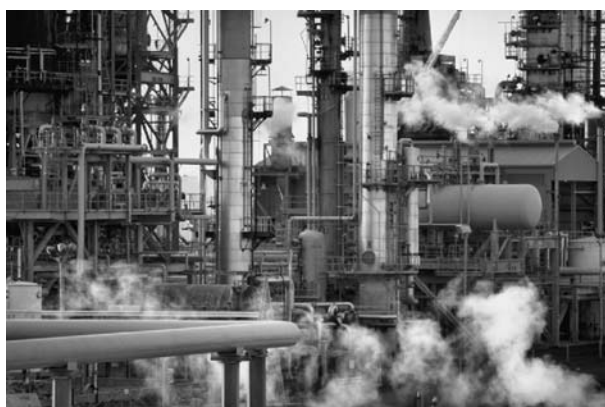
Figure 1: Refineries are composed of a variety of such sophisticated equipment as reactors, towers, heat exchangers, and pipelines.
