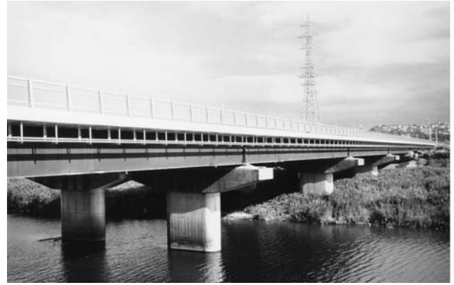
Figure 5: A bridge constructed by using Cu-Ni-Ti type advanced ACR steels and matching filler metals in Japan.
